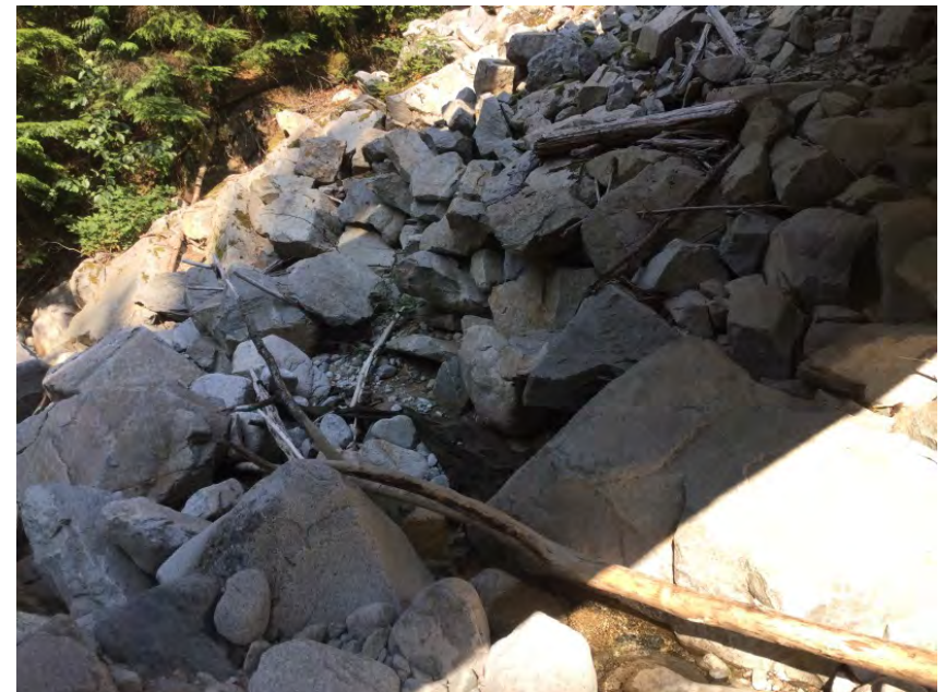
Riprap scour downstream right bank
